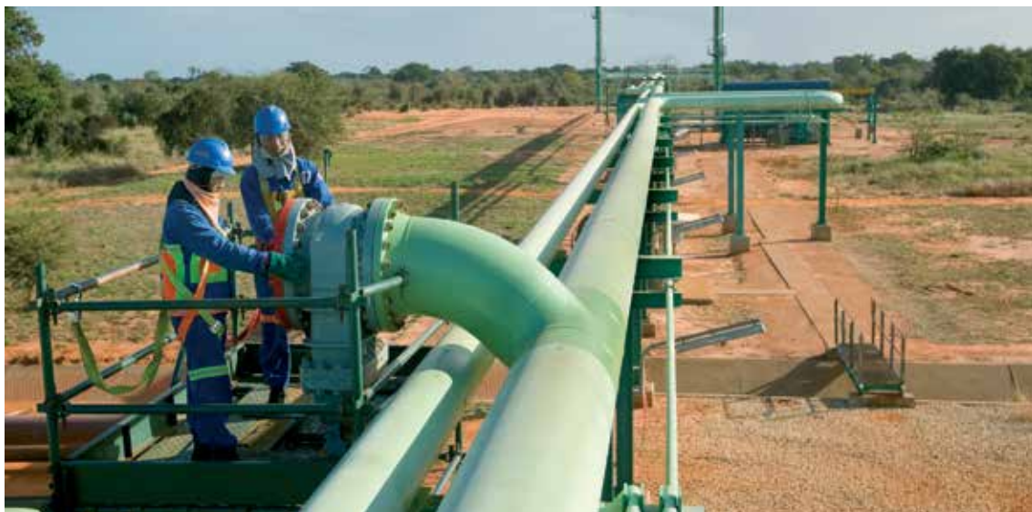
The Sasol gas pipeline in Temane, Mozambique
